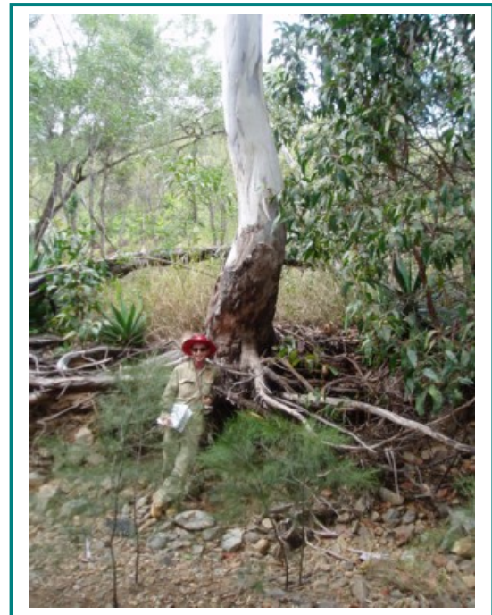
Figure 7. The exposed roots of a Eucalyptus camaldulensis tree on the bank of Gibbs Creek.
